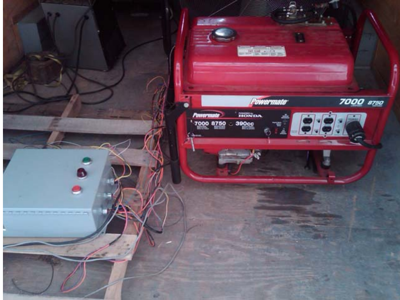
Figure 2.3: EMS equipped Coleman Powermate 7000 Watt generator.
