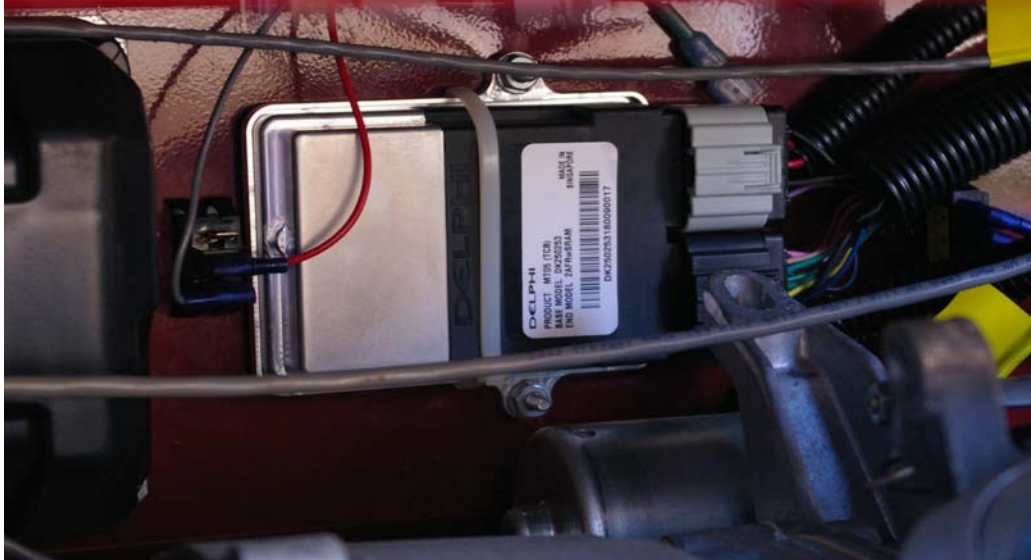
Figure 2.4: Delphi MT05 ECU mounted inside the generator frame [6].
